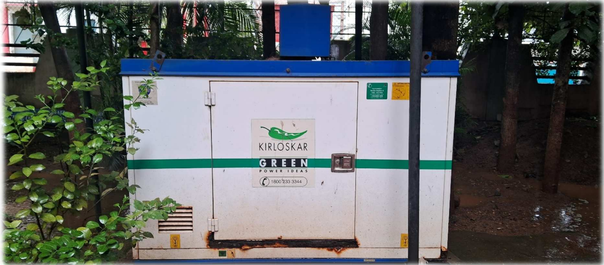
Diesel Generator (alternate source) during power cut
