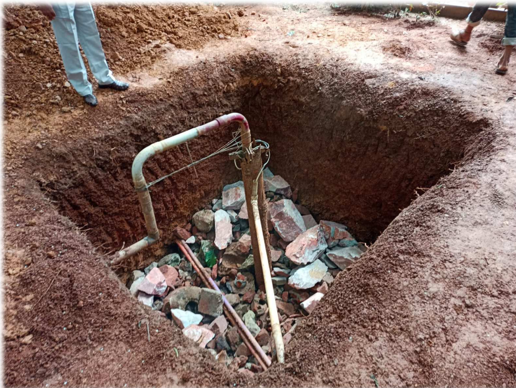
Rainwater harvesting pit around bore well
